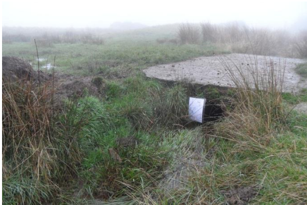
Photo 3.6: Concrete slab bridge (CSB) viewed from upstream, with A4 sheet for scale
